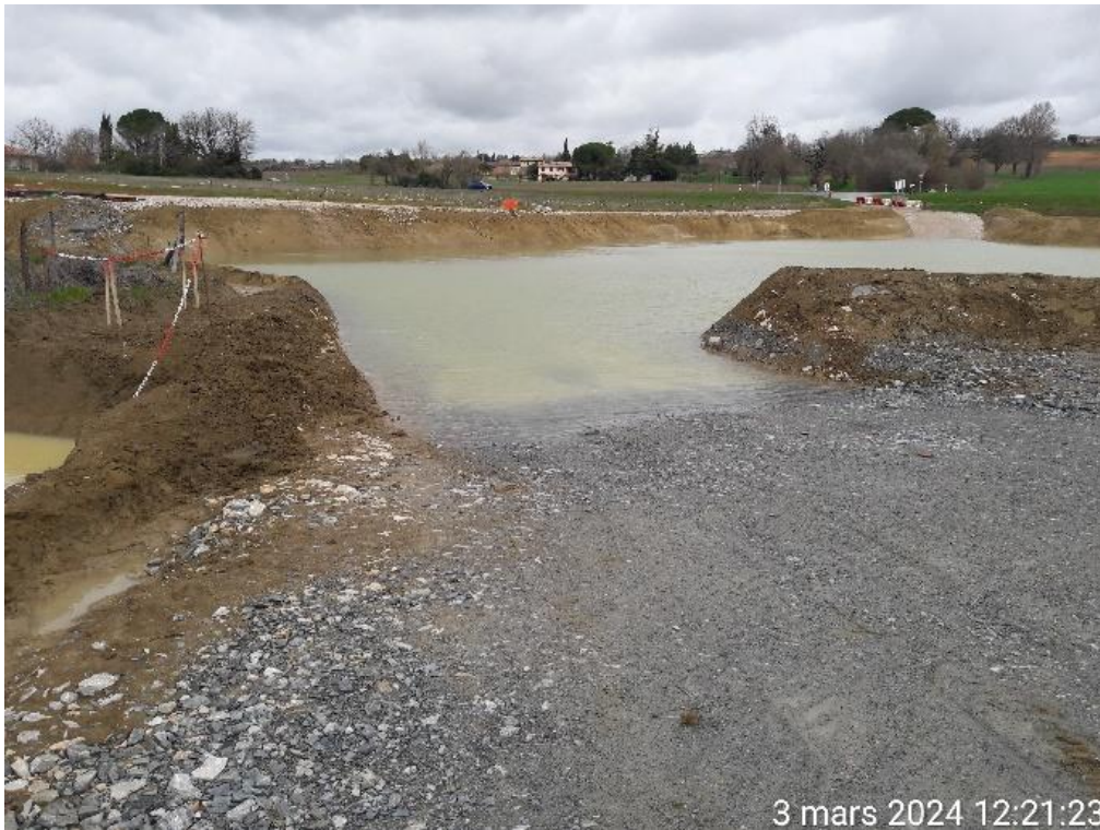
Figure 65: Plateforme inondée MONTCABRIER (81) - Point GPS: 43.612049,1.735803
